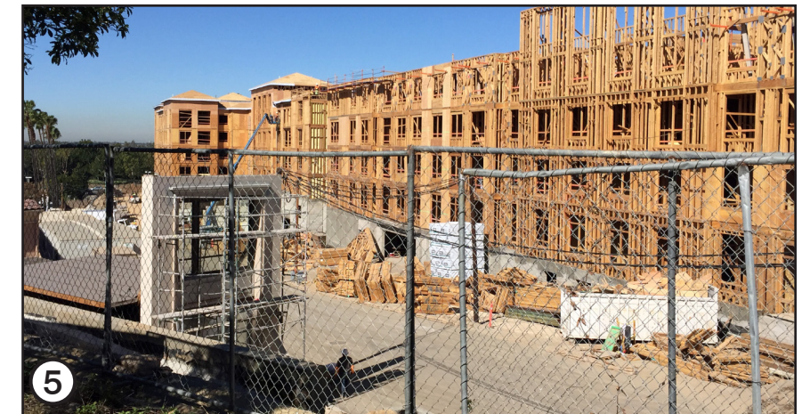
5 View of construction activities for the San Joaquin Plaza residential community north of the project site.
