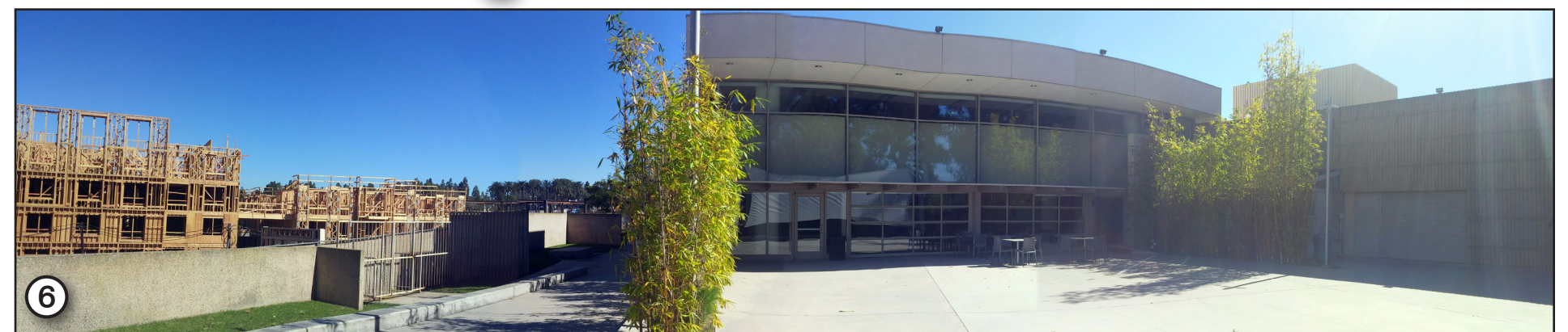
6 Panoramic view of the northwestern building corner and adjacent San Joaquin Plaza residential construction.
