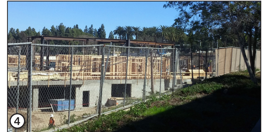
4 View of construction activities for the San Joaquin Plaza residential community north of the project site.
